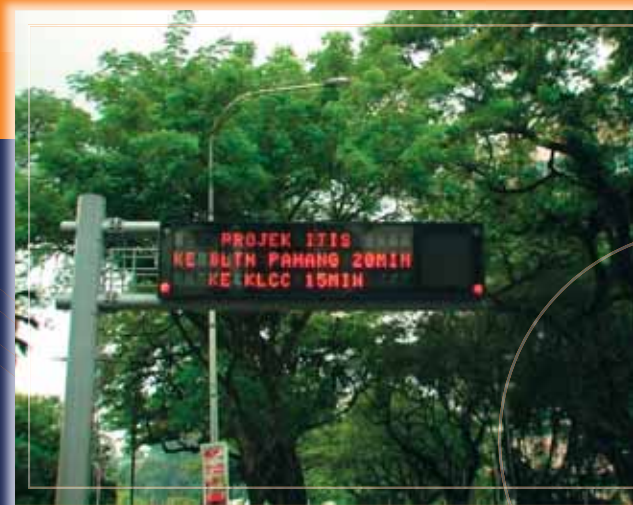
Variable Message Signs - Displaying real-time traffic information
